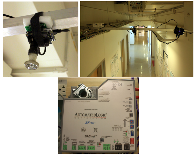
Figure 1. The upper left image shows an Imote with an IMB400 camera and a fisheye lens. The upper right shows several cameras deployed in a hallway. The bottom image shows a ventilation damper actuator made by Automated Logic.
